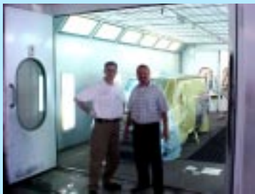
Paint shop manager, Sarkis Kalechian and assistant shop manager Kevin Daghla in heated downdraft drive-through spray booth
